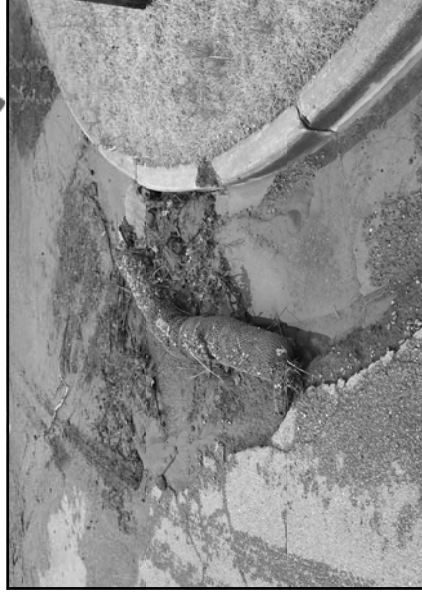
The inlet protection above was intentionally moved during a storm event causing a serious discharge of sediment into the stormdrain
